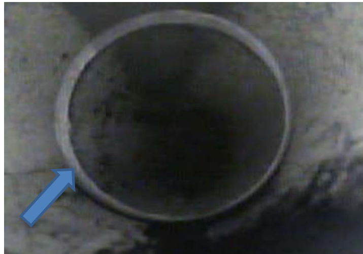
Figure 5: Break Identified in the Supply Pipe
